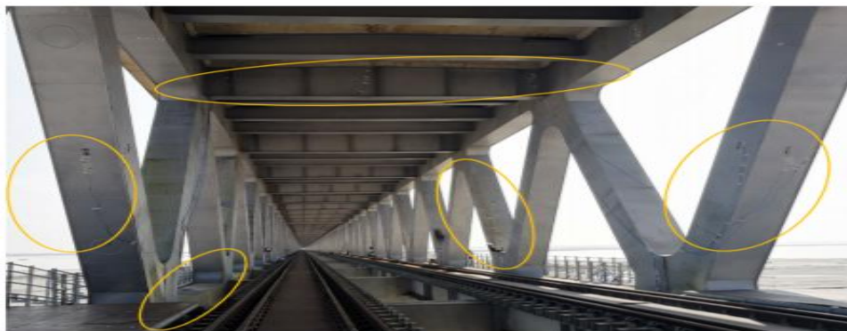
Strain gauges and thermocouple installed on bridge
